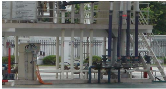
Our Batch Controllers were installed at such petroleum trucks terminals
